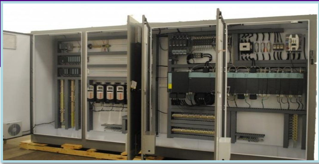
Automatic Control System
